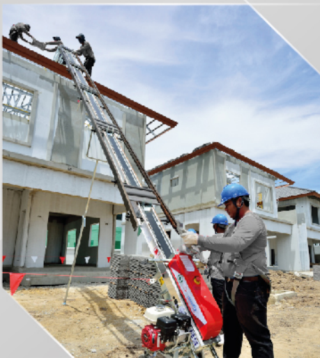
The tiles will be transported by the conveyor belt for safety and process time reduction.
